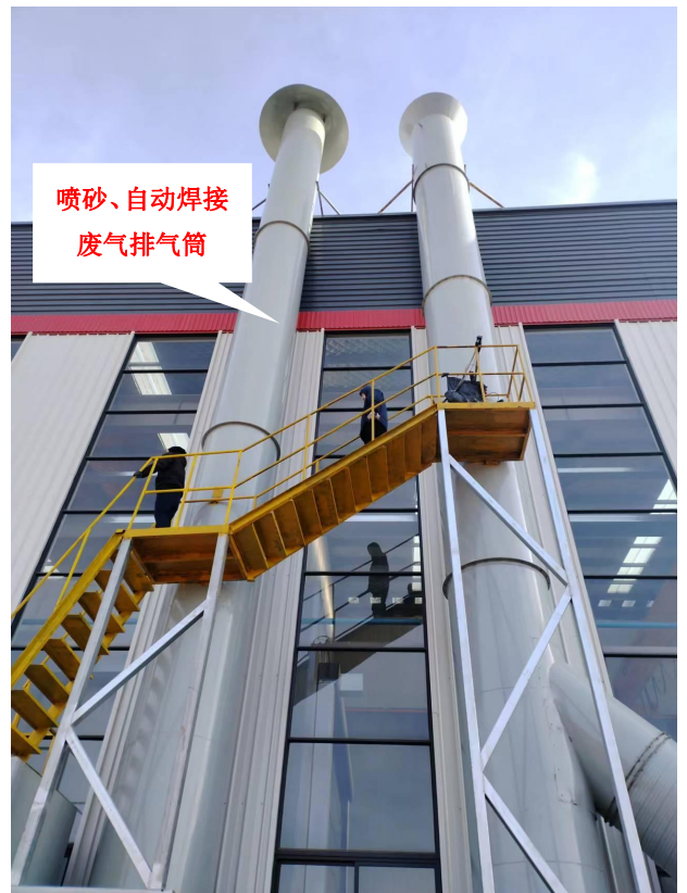
喷砂、自动焊接滤筒除尘器及排气筒 DA001
